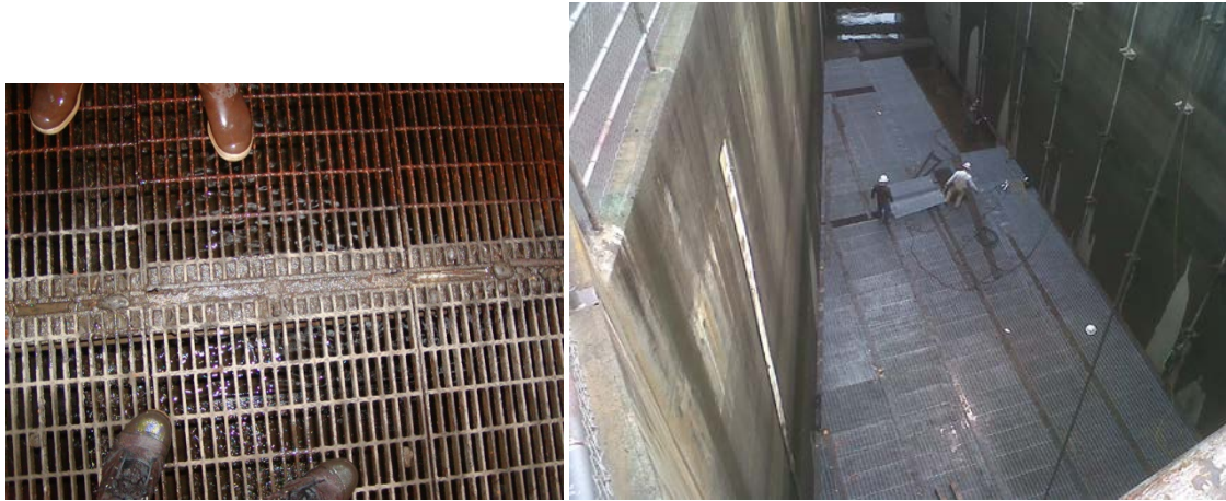
Figure 1: Horizontally-oriented AWS diffuser grating. [Photo credit: Robert Cordie, U.S. Army Corps of Engineers].
